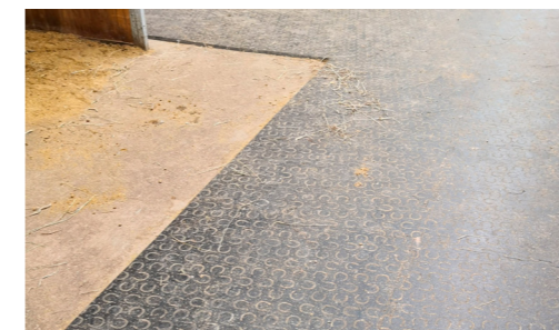
rubber floor in stable to protect hooves and facilitate cleaning
