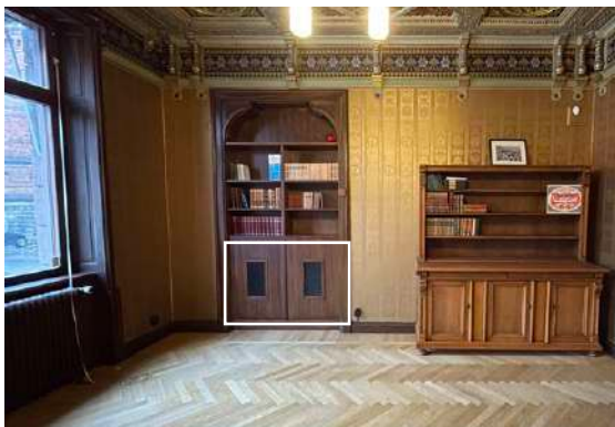
Image 44. West wall, with the hidden ventilation in the built-in wooden bookshelves. (white rectangle).
