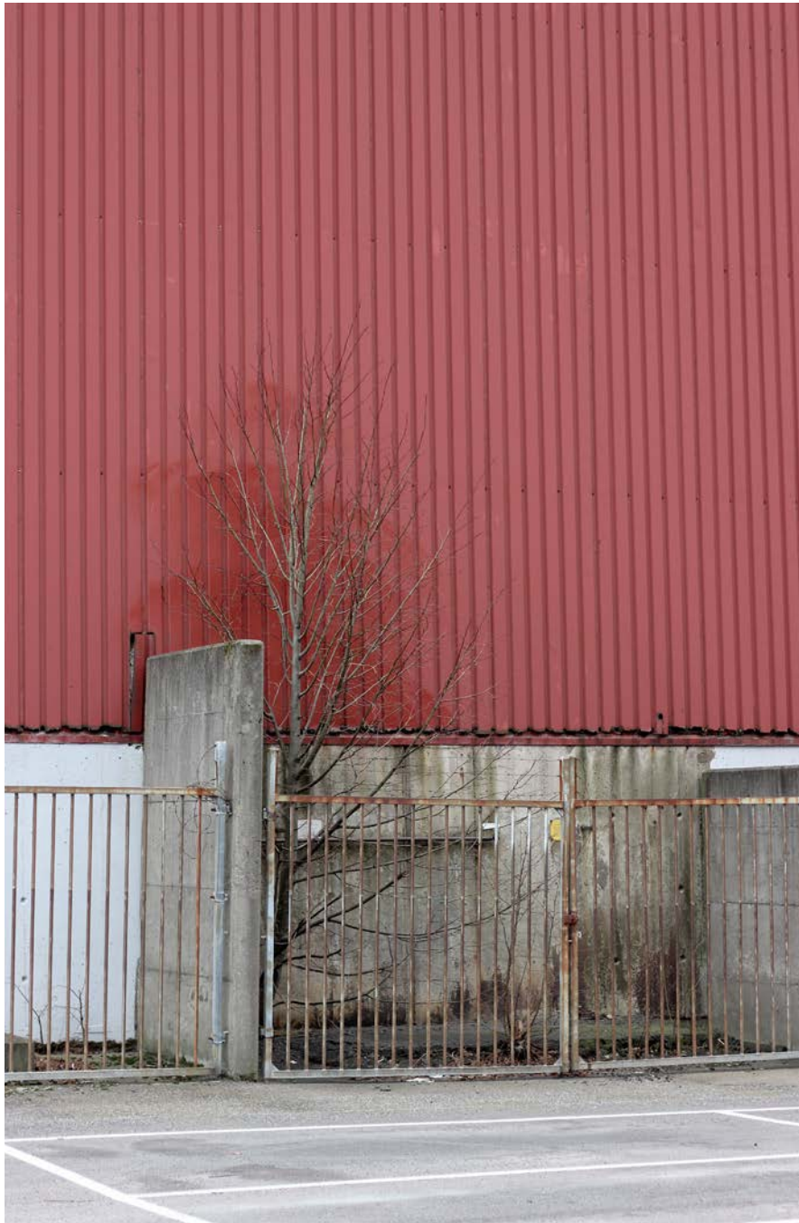
An encapsulated tree growing along the facade.
