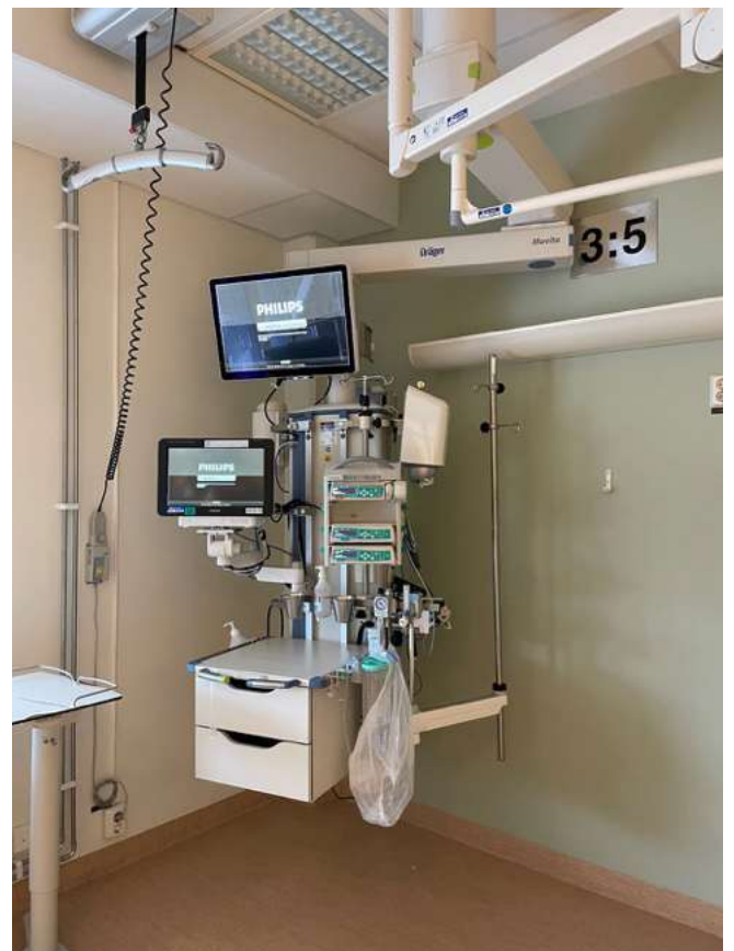
Medical equipments attached to the ceiling in care room two and three
