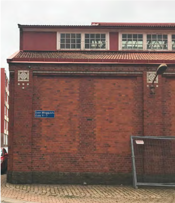
bricked up windows
