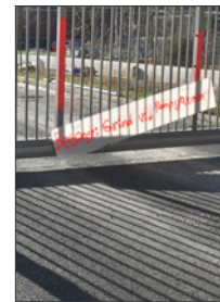
8 (Fig. 35) Warning for concrete gate.
