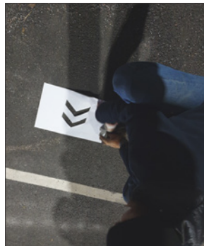
Fig. 84. Marking the ground with an arrow pointing towards the stairs.
