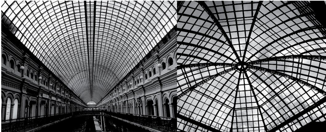
Figure 6. The Roof of the Upper Trading Rows in Moscow and the central Dome portion (1890).
