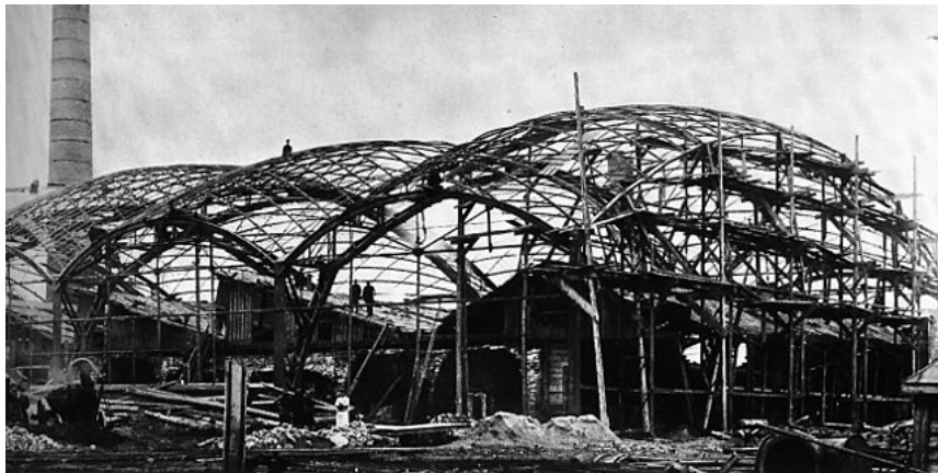
Figure 7. The world's first doubly curved steel gridshell exhibition hall under construction in Vyksa near Nizhny Novgorod, for the All-Russia Industrial (1896).
