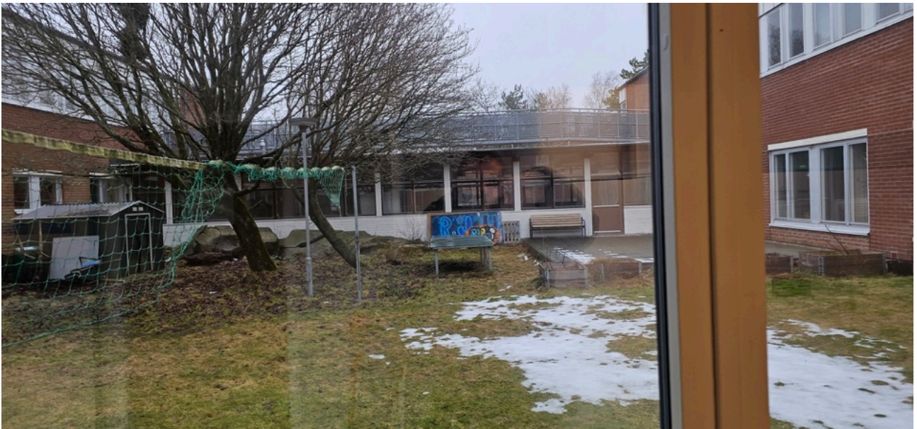
Figure 35a. Picture of the former youth center, Tyrolen. It is not used due to a mold infection in the ceiling.
