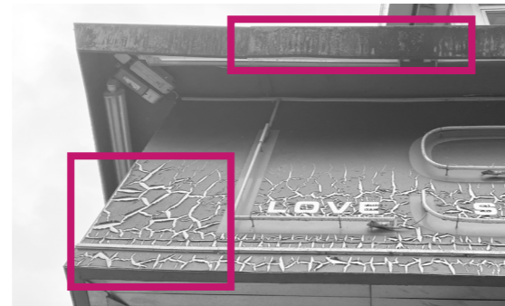
Fig. 22. stains on facade
