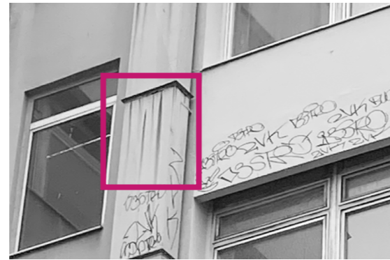
Fig. 21. stains on facade
