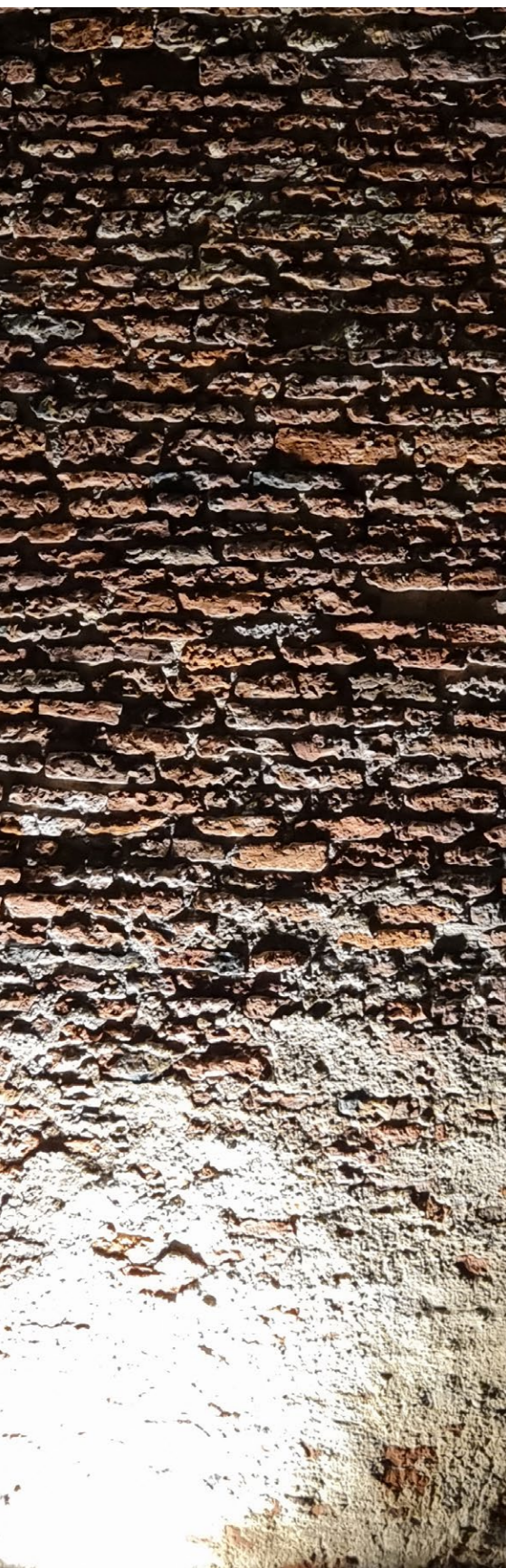
The photo highlights the intricate texture of a brick wall within the settlement, showcasing the unique craftsmanship and strength embedded in the community's infrastructure. (Photo by the authors)
