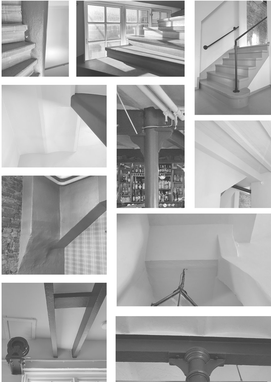
Several remenants from the inventory worthy of being kept and/or being protected by the protection act
