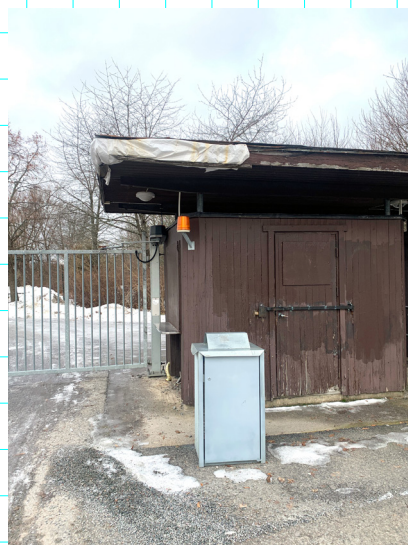
4a. The gate to the sports field Not in its intended use, a barrier and a storage. Some repairs and attentions to keep it as it was.
