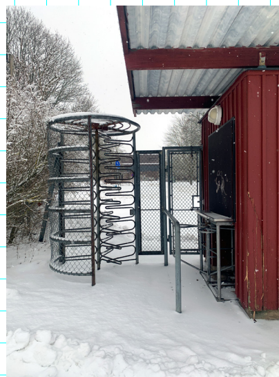
4b. The gate to the sports field 2 Not in its intended use, a barrier and a storage. Working as a notice board. Some repairs and attentions to keep it as it was.
