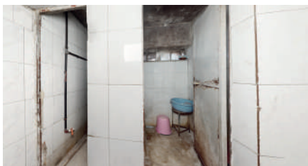
Figure 21. Current condition of the guard rooms in the basement level. Source: Adapted by the author from Syrian Prisons Museum.
