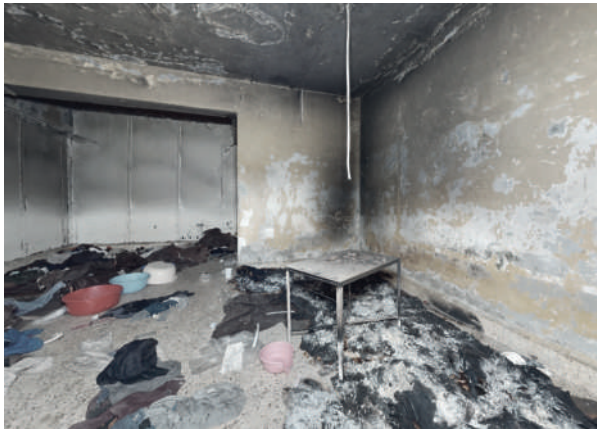
Figure 35. Traces of fire in “Cell 1 – A Right”, second floor. Source: Adapted from Syrian Prisons Museum.
