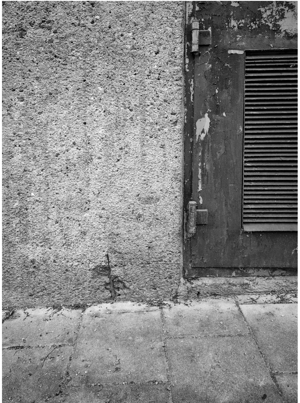
Fig.40 Damage of the reinforced bars, the concrete coating and deterioration of doors.
