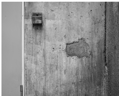
Fig. 25 Concrete surface deteriorations, Hornsbruksgatan 4.   In es Romy
