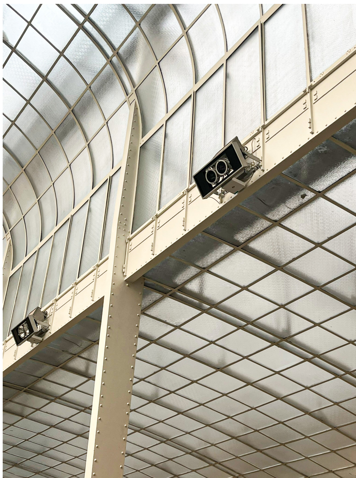
Figure 2: Glass roof of the Grand Cashier Hall with newly added light element during renovation, observing the space below. Author's photograph.
