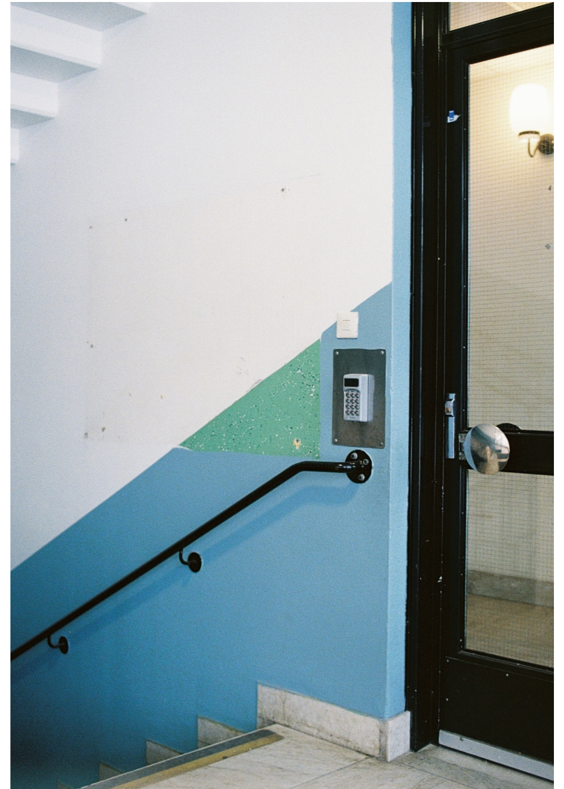
TRACE OF FORMER STAIRCASE WALLPAINT
