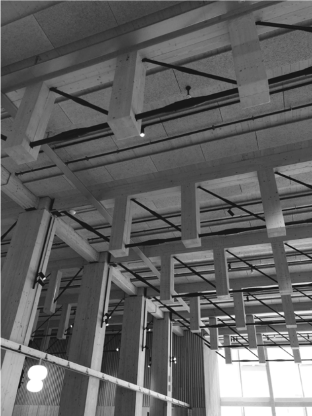
Figure 06. Sara Kulturhus: Wooden roof and black steel details. (Palmqvist, 2020). Published with permission.
