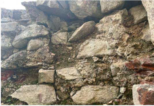
Fig. 40 Section of collapsed wall. Photo by author.
