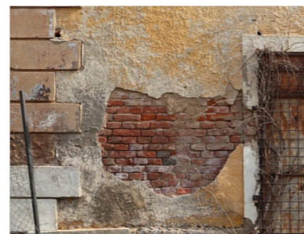
Figure 54: Non-structural decay of the barracks' external painted lime render
