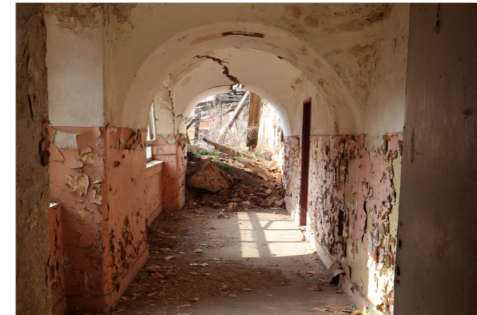
Figure 51: Figure X: A corridor leading to a collapsed section of wall and roof
