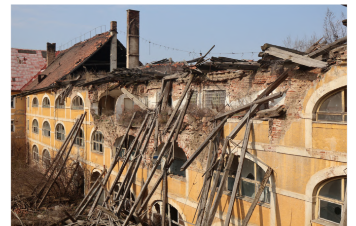
Figure 52: A collapsed section of second floor corridor wall and roof. The Dresden Barracks is in a constant state of deterioration
