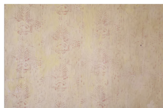
Figure 53: Some second floor rooms in the barracks are decorated with hand-painted wallpaper, put up during the Czechoslovak army's occupation after WWII
