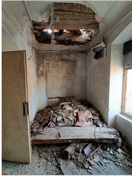
Figure 67: The former soldiers' chapel; both floor and ceiling will be removed to create a triple-height communal spiritual space
