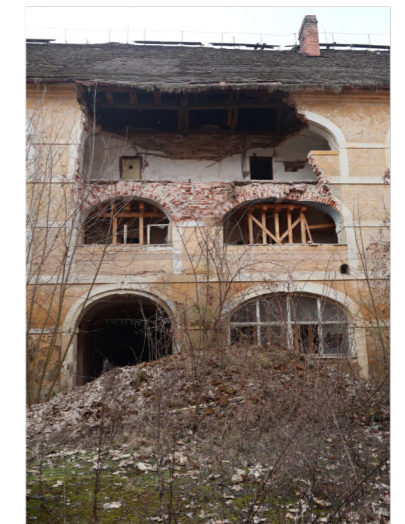
Figure 56: Further collapsed wall sections in the proposed sculpture garden
