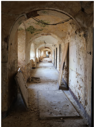
Figure 38: The corridors in the Dresden Barracks are crumbling and marked with layers upon layers of peeling paint
