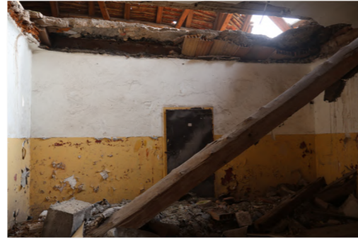
Figure 39: The ceilings of many spaces on the second have collapsed, revealing the roofspace above
