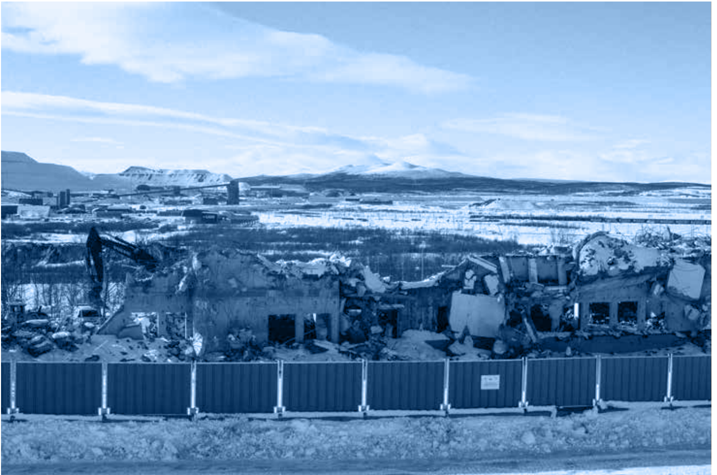
Fig. 50 Demolition of old Kiruna, while iron ore mining continues in the background
