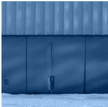
Fig. 44 Crack in Plinth (Old Kiruna), 2026
