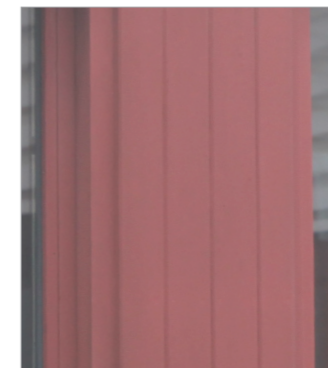
Material: Wood Category: 02 Envelope Reuse Potential: Easy
