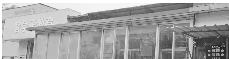
Figure 18. The photos show the existing issues of the community building.
